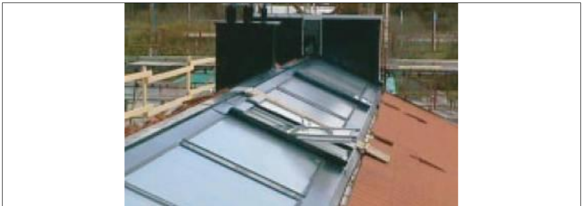
Figure 5.4: Solar collectors and roof windows at Lindas Passive House Project
