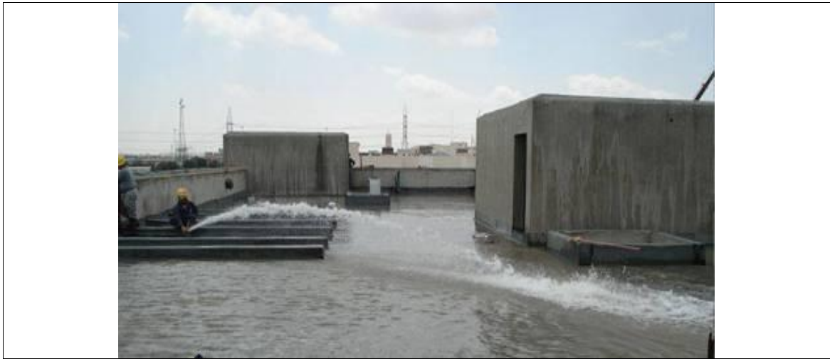
Figure 4.20: The process of inspecting waterproof with submersion method Source: (The Engineer Site for Construction and Decoration, 2009)
