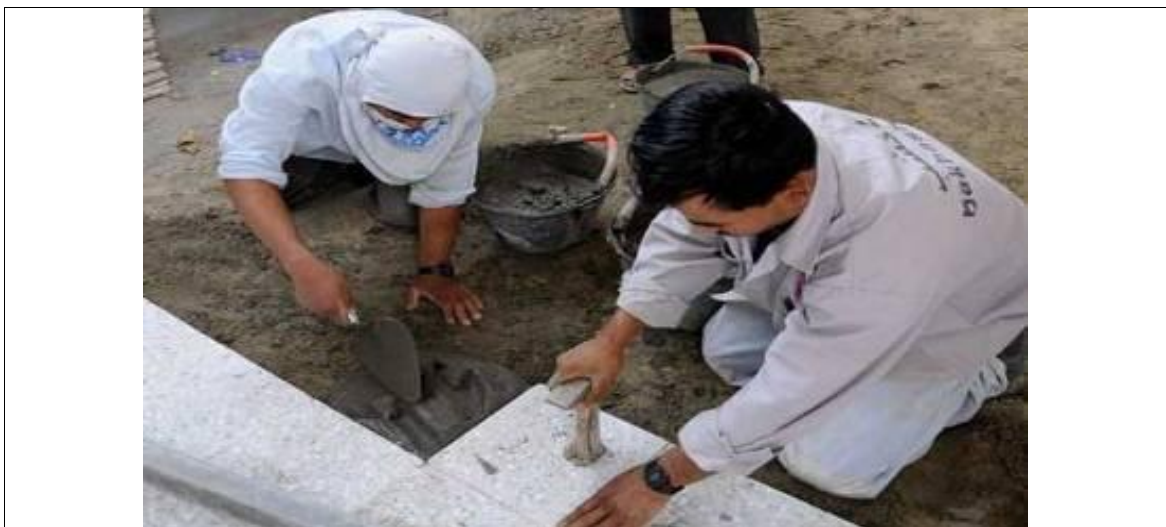
Figure 4.21: The process of installing tiles over the protective concrete layer Source: (The Engineer Site for Construction and Decoration, 2009)
