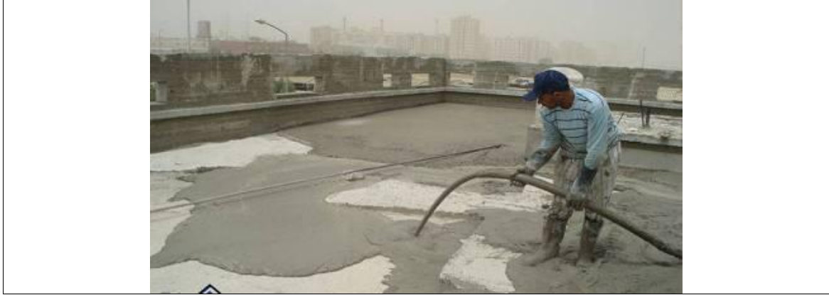
Figure 4.18: The process of pouring a layer of foamed concrete on the roof
